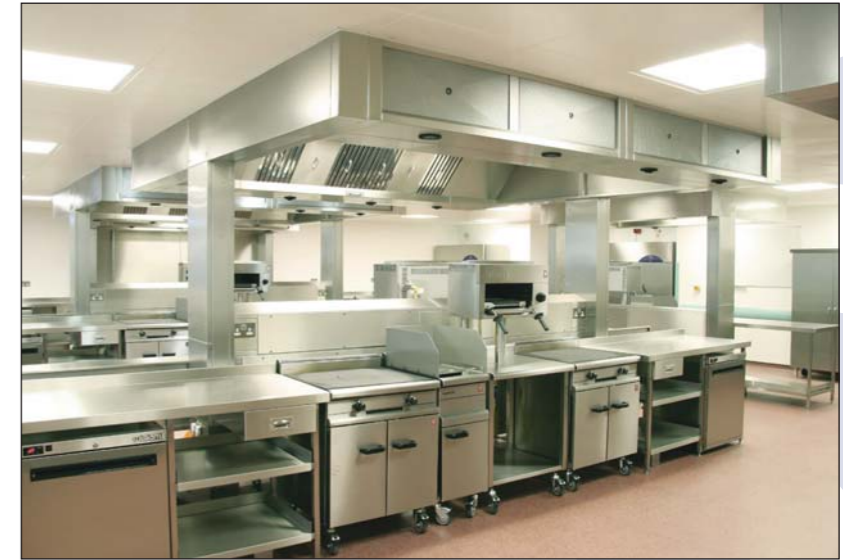
One of the largest kitchen ventilation projects in the world delivered on time and on budget
